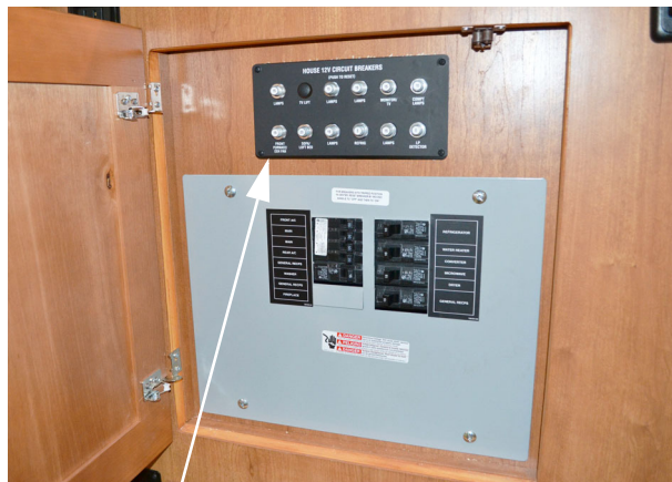
House 12-Volt Circuit Breakers
