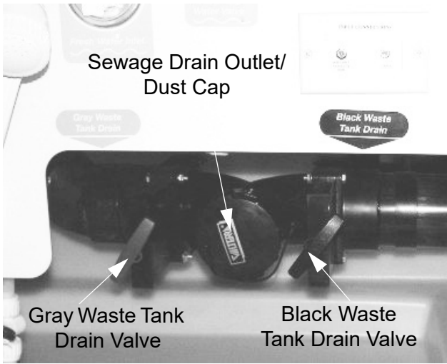
Holding Tank Drain Valves (Located in water service center) -Typical View
